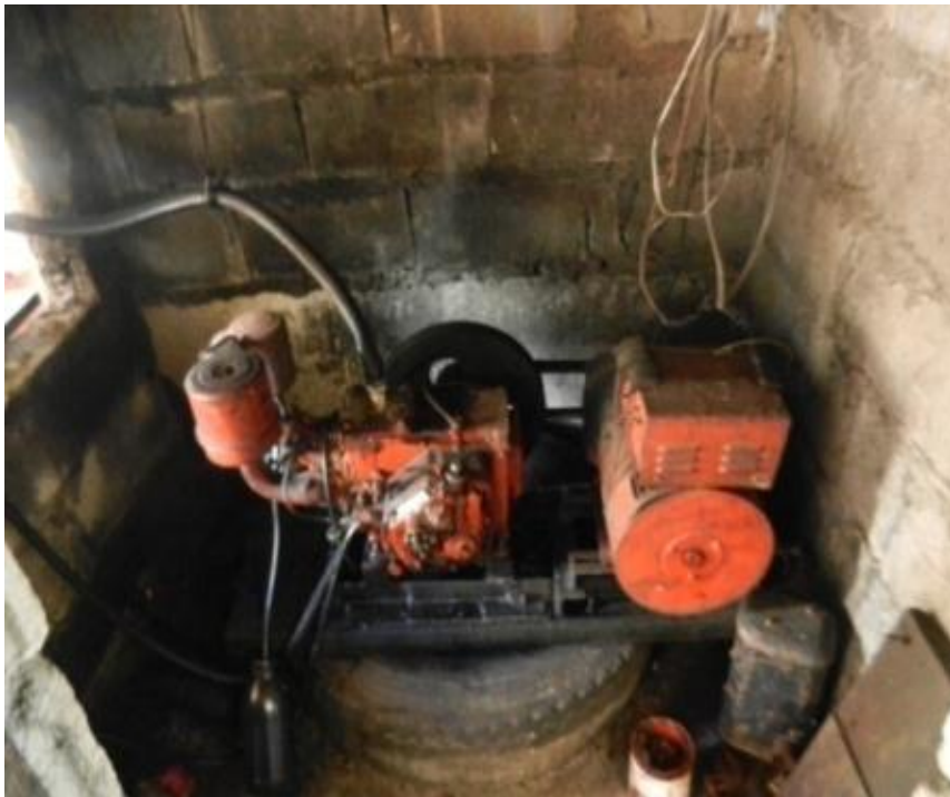
A typical Diesel Genset
